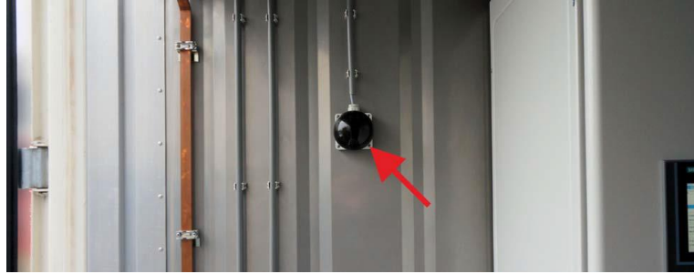
Process Stop Button in ESI Room
